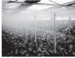
Overhead Irrigation System
